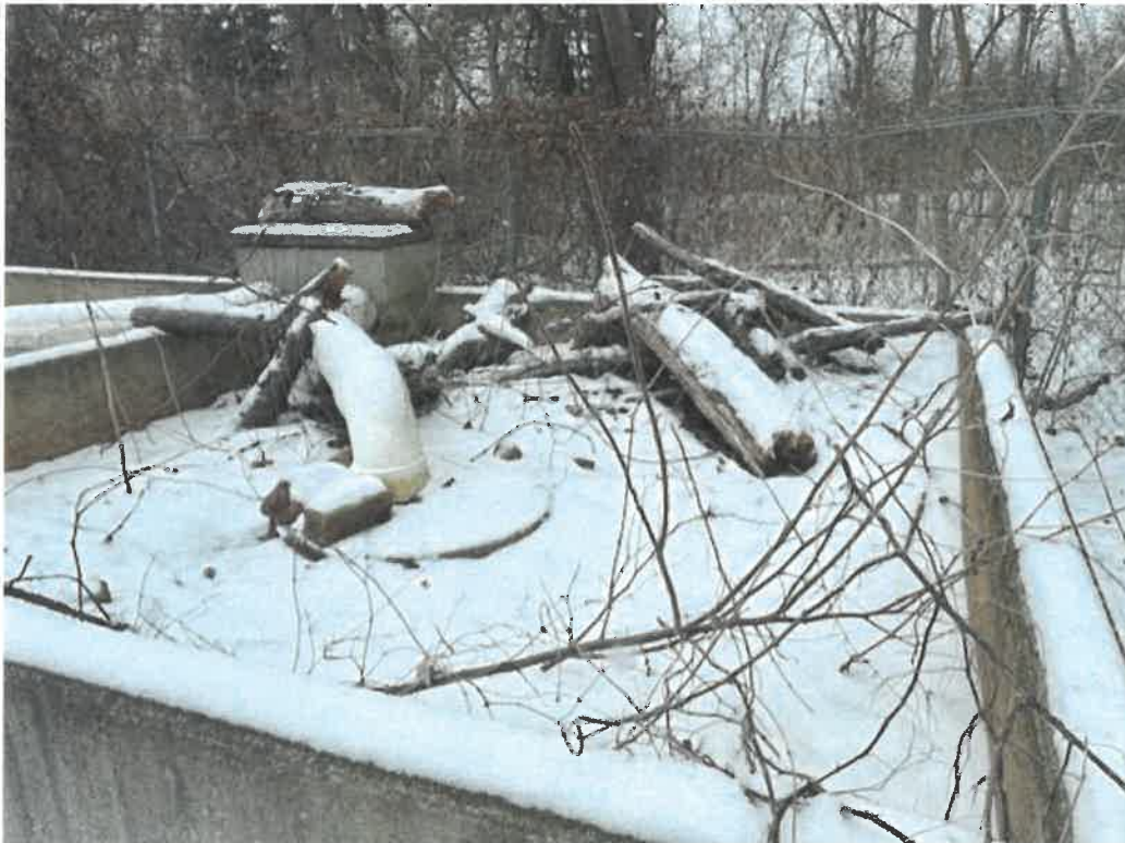
Branches and wood debris on sand filters.
