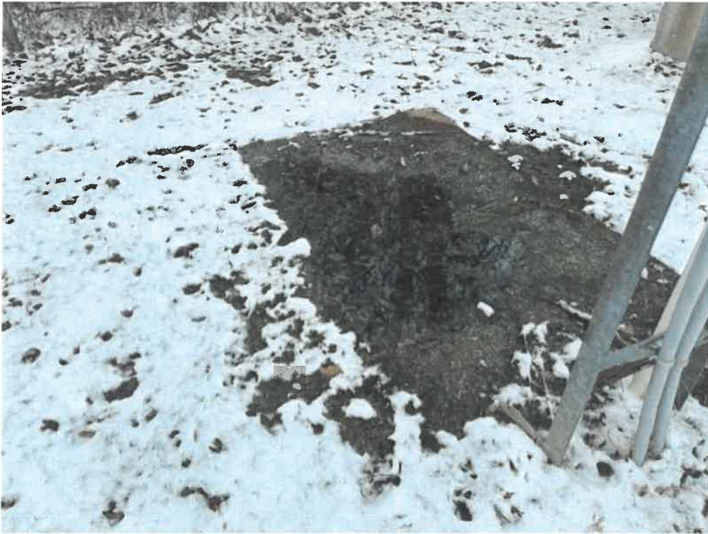
Ponding effluent at pump tank.
