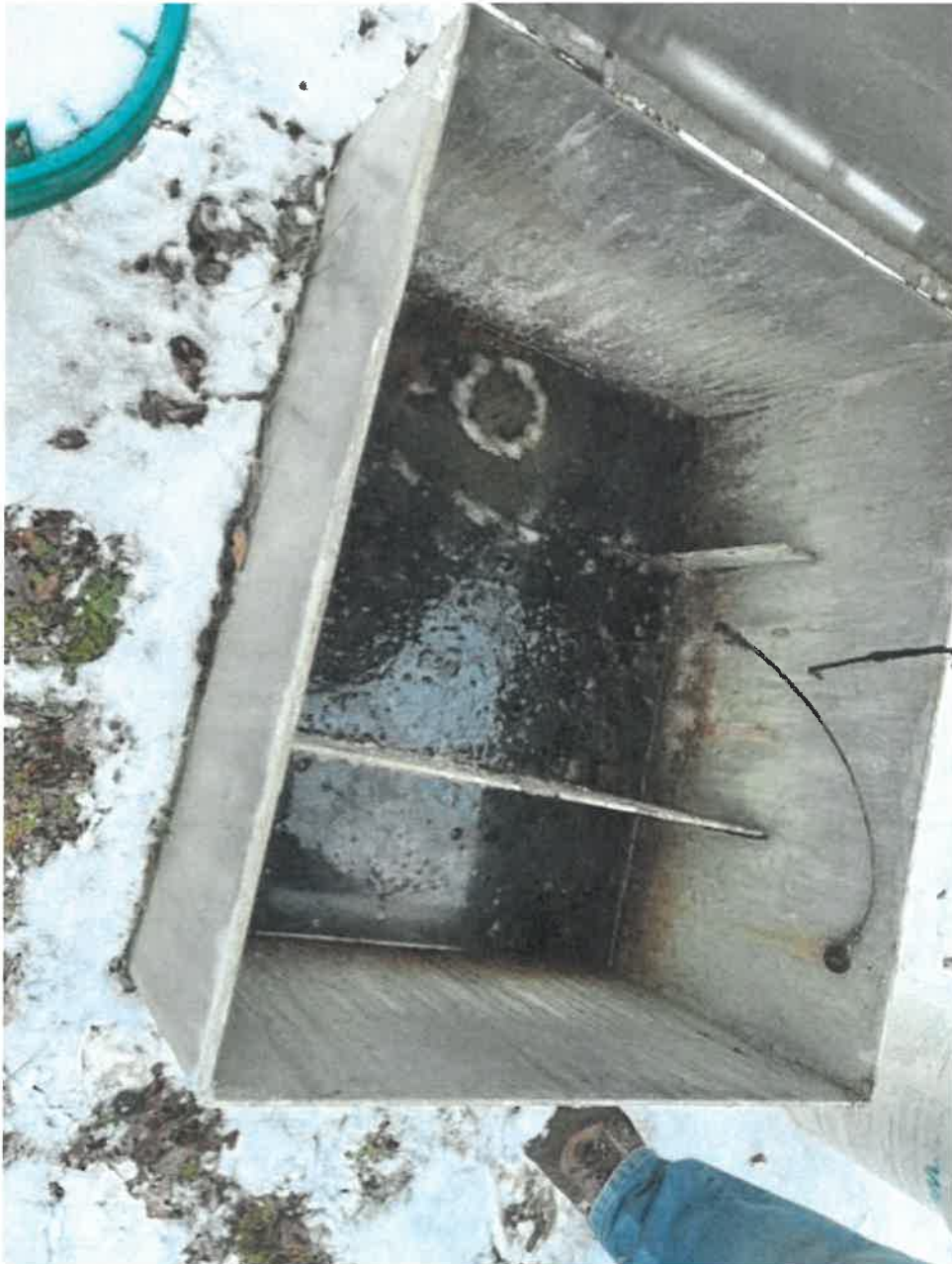
Overly full EQ tank.
