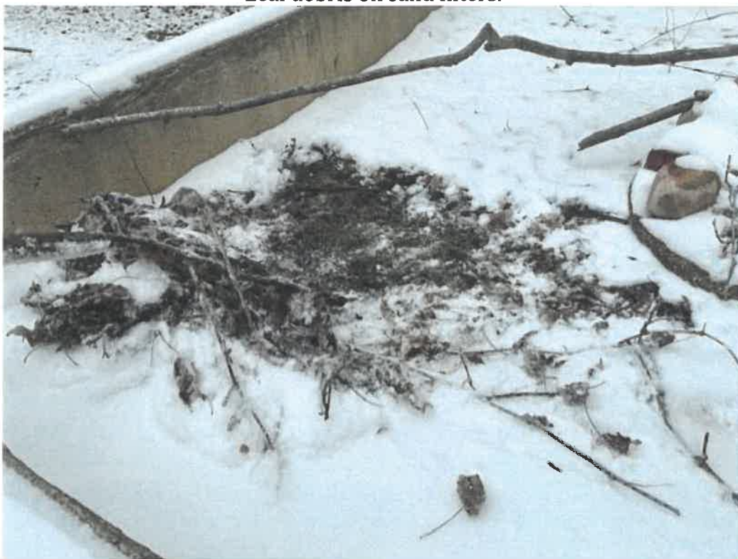
Leaf debris on sand filters.
